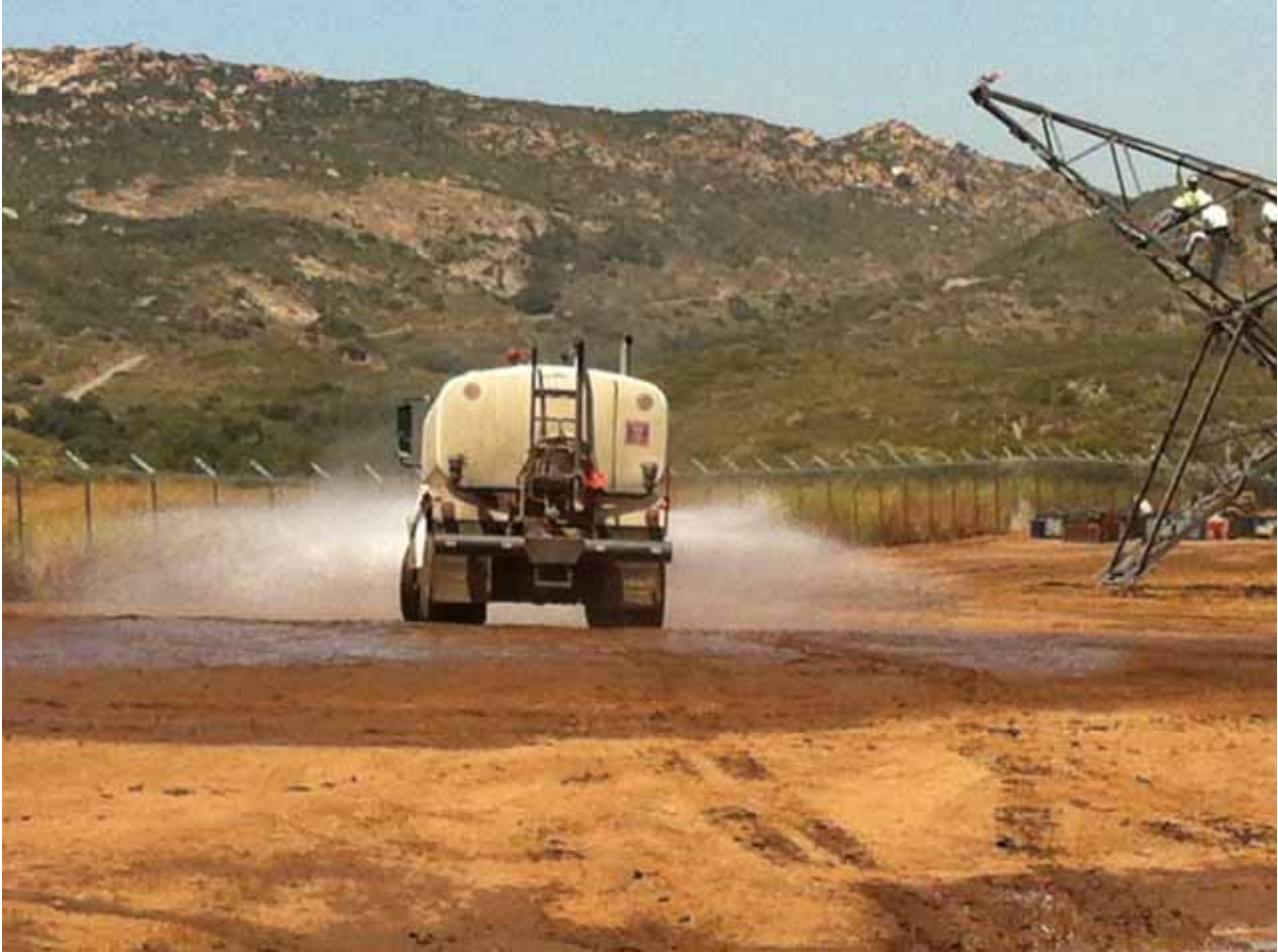
Reclaimed water being used at SWAT Yard ( Photo courtesy of Mike Vader )
